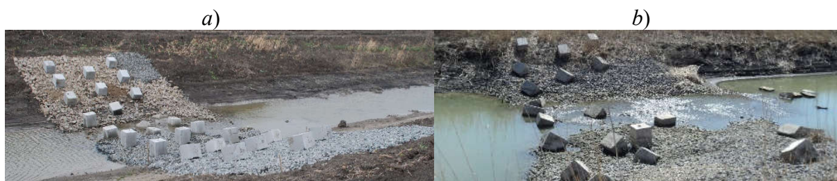
Figure 3 – View of the arrangement of elements of enhanced roughness in the fish passage and spawning channel tract
